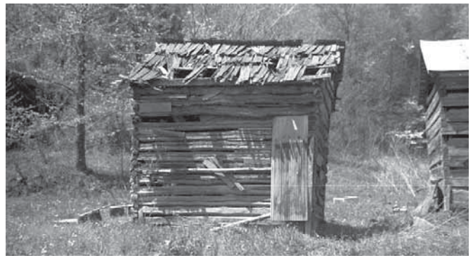
Figure 5: When Shell first arrived on his farm in Leslie County, a small abandoned cabin was already there. According to Shell, his family lived in this makeshift cabin with a single door and no windows until the larger hewn log cabin could be built. The edge of the larger permanent cabin can be seen behind and to the right of the small cabin. Later accounts said the smaller cabin was a smoke house, and the main cabin was already there when Shell arrived about 1867. This picture was taken in 1975. Courtesy Kentucky Heritage Council, Frankfort, Kentucky
